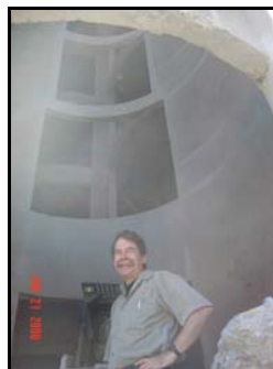
Architect Mike Malinowski inside one of the Globe Mills' concrete silos under construction for new housing units
